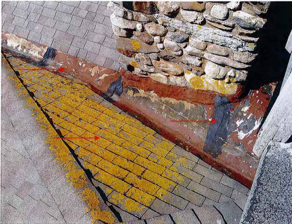
Photo 3: Roof failure. Patches and layers of flashing reveal an attempt to correct the problem originating from when the building was enlarged and the tower constructed. The building was not engineered for the long-term success and functionality of the roof, which has failed because of inadequate water drainage, and has resulted in water penetration in the interior. A new, engineered roofing system will be installed.
