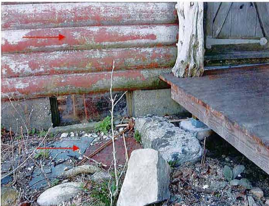
Photo 14: Historic paint and debris. The exterior of the building was originally painted red. A scientific paint analysis will be undertaken to determine the precise shade of red that was used and the building will be repainted accordingly. All debris on site will be removed and recycled.
