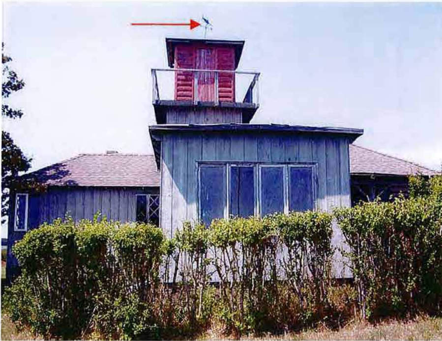
Photo 13: Historic weathervane is non-functioning. The weathervane will be restored to functioning and weatherproofed.
